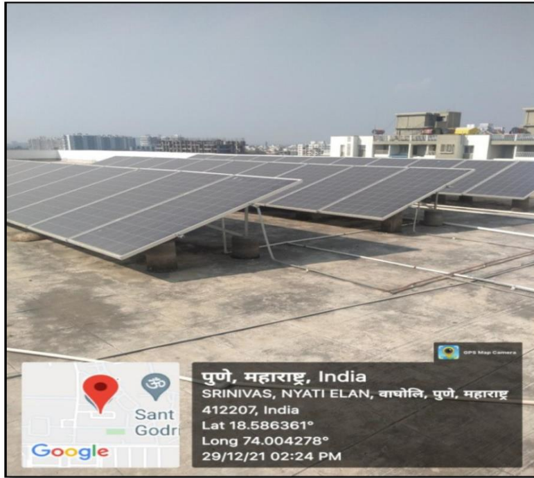
Roof top Solar System
