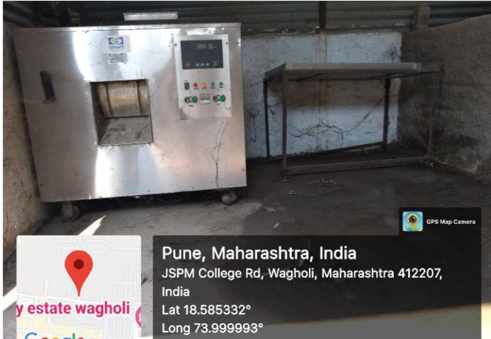
Organic Converter Unit
