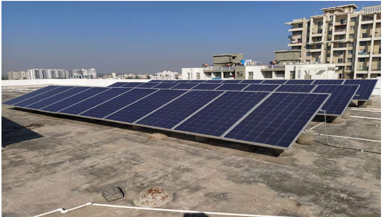
Photo 1: Solar Panel Installed
