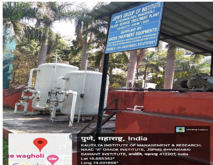
Sewage Treatment Plant
