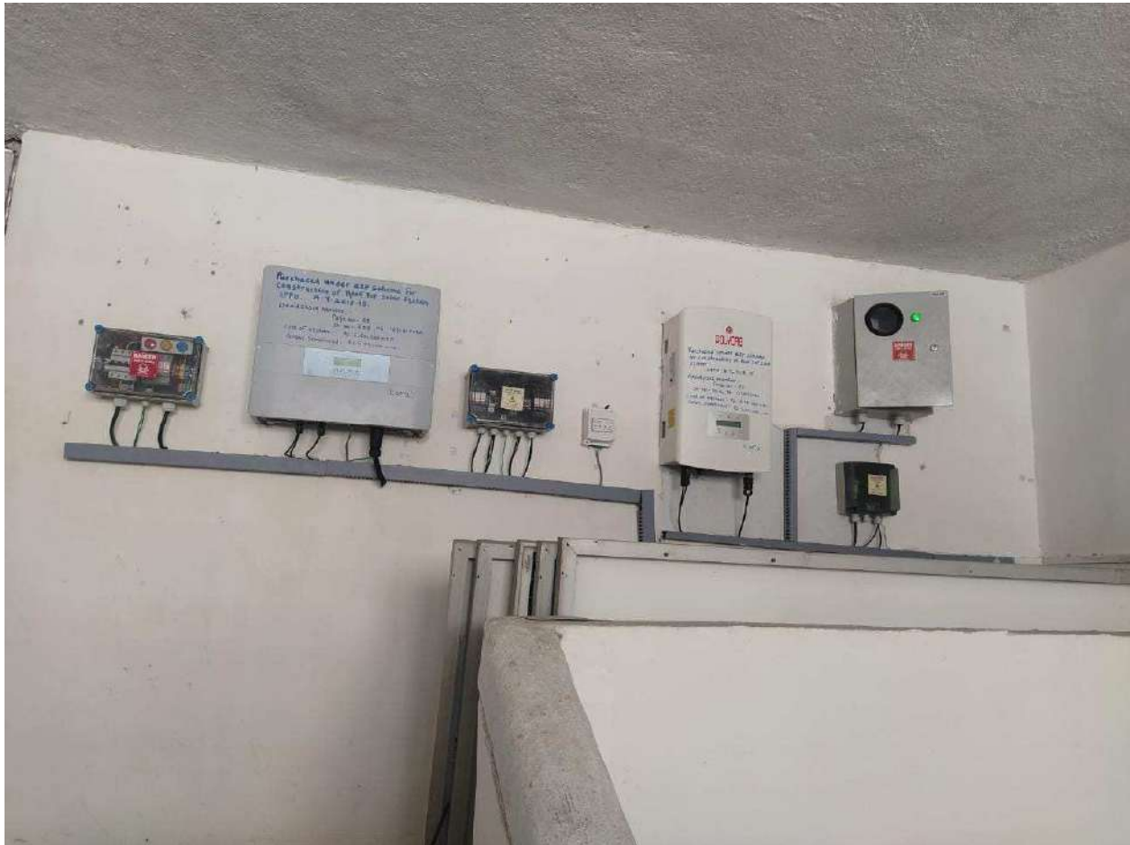
Photo 3- Solar Panel Details Installed
